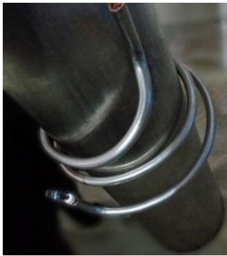
Figure 9 Electrical resistance installation
