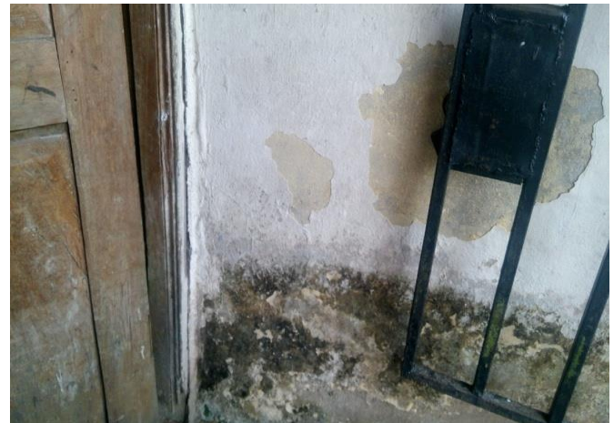
Plate 3.2: Picture showing decaying wooden door due to moisture and flooding on a property in study area.
