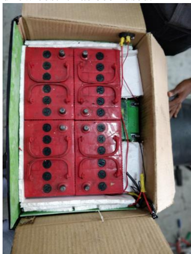
Fig. 9: Lead acid battery
