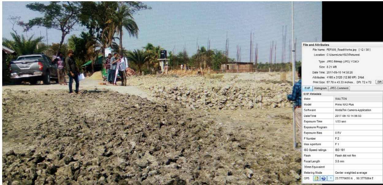
Figure: 10, Work component submission by FRE with data and timestamp with GPS Code
