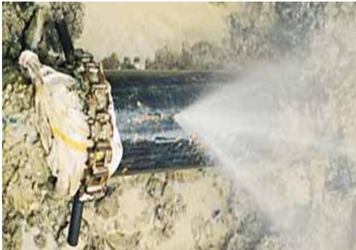
Fig.2 Small Leak on Cast Iron Water Main
