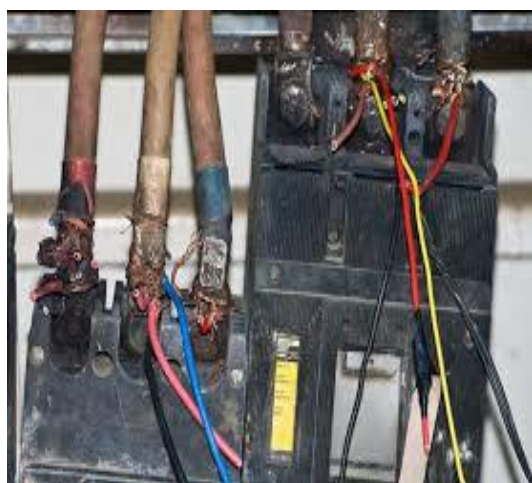
Figure 5: Electricity bypassing by customers in Kisumu Source: Field data (2019)
