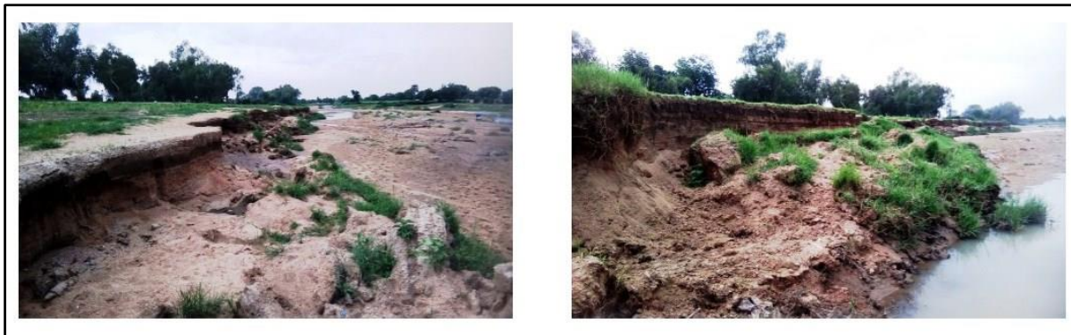
Plates 3 and 4: Eminences of channel banks failure at concave (outside) banks
