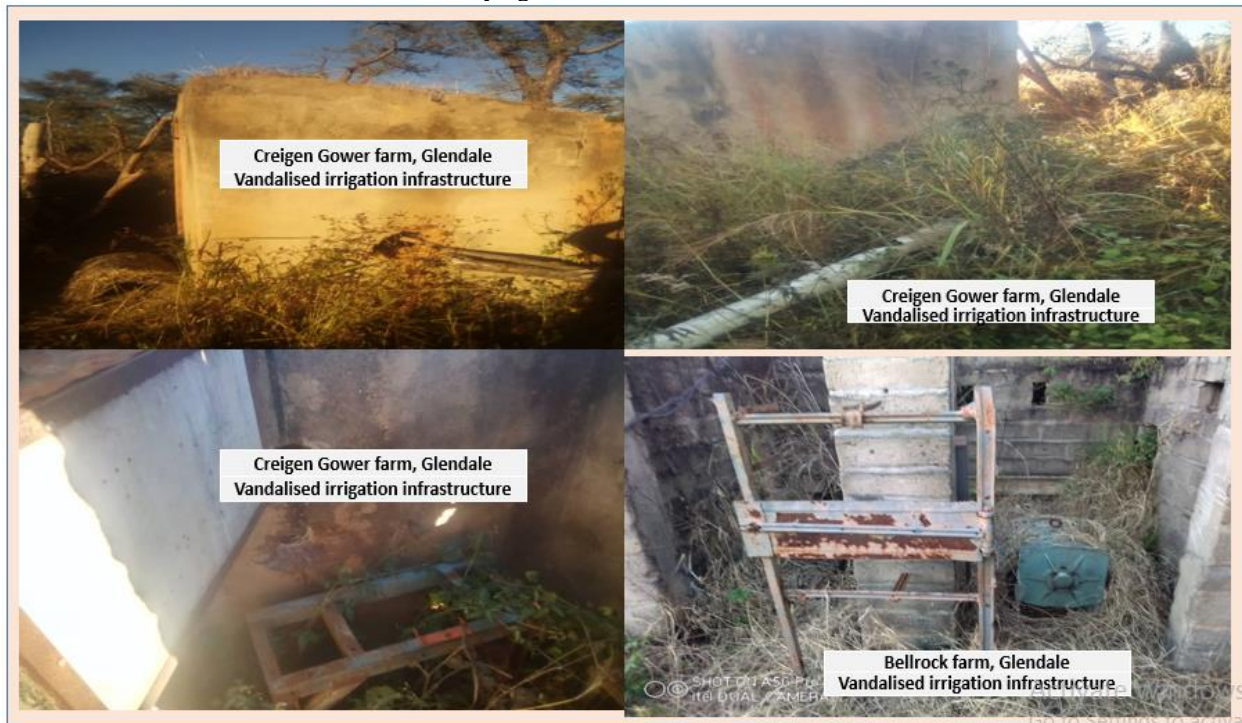
Figure 3: Vandalised irrigation infrastructure Source: primary data, (2021)
