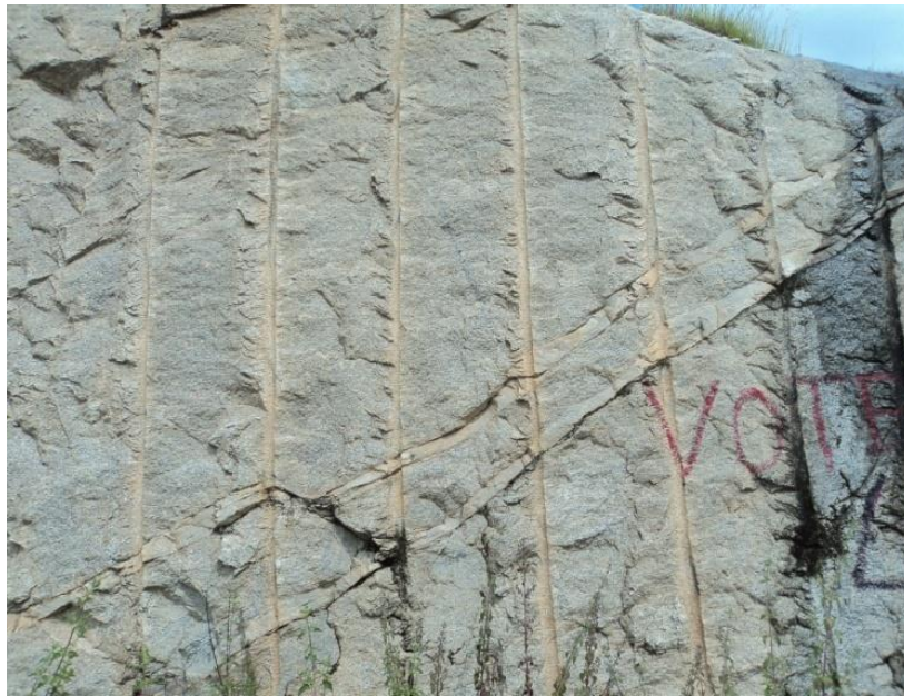
Plate 5: Joint on granite rock cut across along Sarki pawa road
