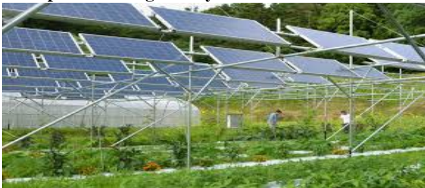
Plate 3, Image of solar operated irrigation systems.
