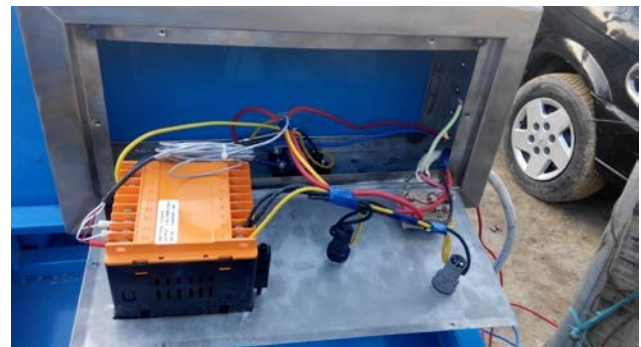
Figure 13: Temperature Controller box set up.
