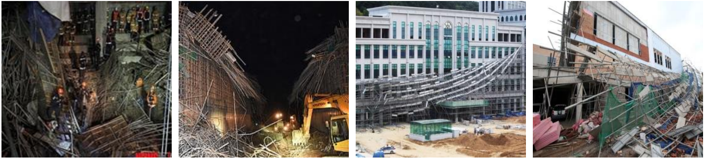
Fig. 1. Failures induced by use of inappropriate temporary equipments and materials: (a) Nengsumulcheon Bridge in Yongin city; (b) Sadang Complex Gymnasium in Seoul city; (c) University Building in Cheonan City; (d) New Construction Sites in Pohang City
