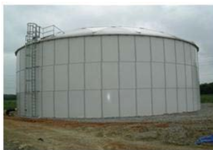
Figure 4: Fire protection water storage tank.
