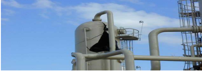
Fig. 2. Failure of pressure vessel during hydro Test.
