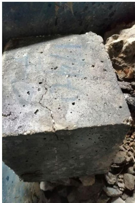
Plate 2: Fine cracks indicating failure
