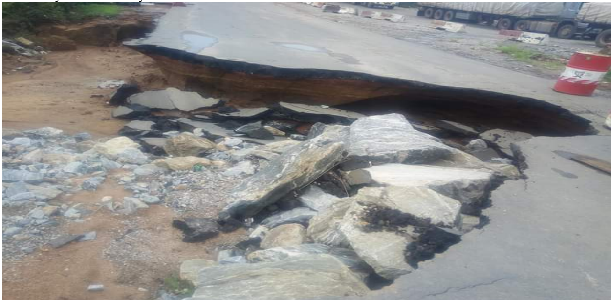
Fig 2: A failed portion of road under study
