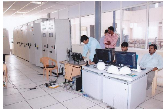
Fig 1: Entire view of DCS Room.
