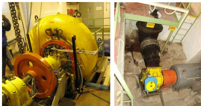
Figure 4:View of turbines HC1 Francis (left) and HC2 Banki (right)
