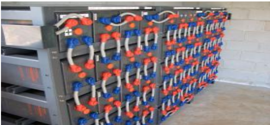
Figure shows Battery Bank
