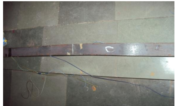
Fig.12 Lateral Torsional Buckling of ISMB 150
