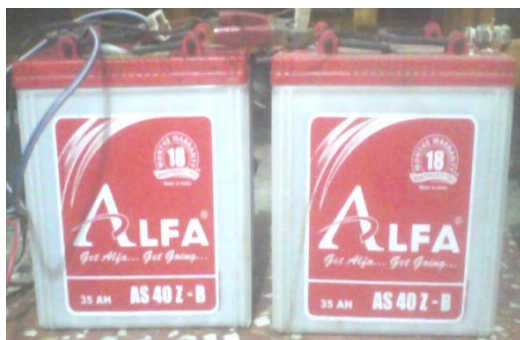
Fig 8: Lead Acid Battery
