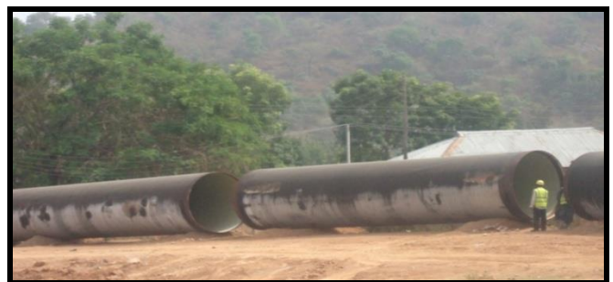
Plate VI: The 75 Km Long, 3m Inner Diameter Transfer Pipes Azara - Jere irrigation scheme
